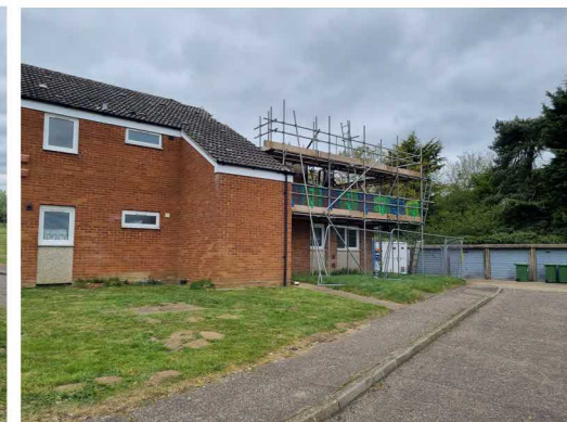
Fire damaged flats and dilapidated garages beyond
