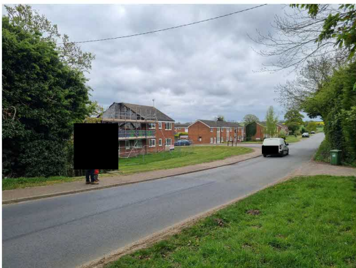
Looking south along the Fakenham Road, with fire damaged flats and site on the left
