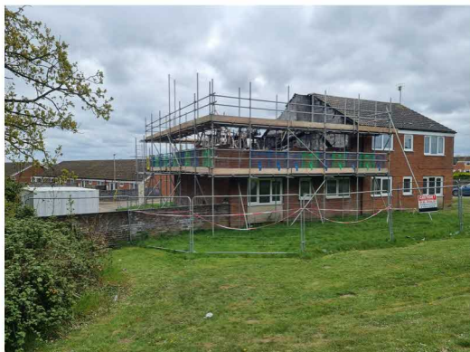
Fire damaged flats on the site
